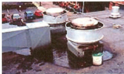
Roof Without Grease Guard Protection
